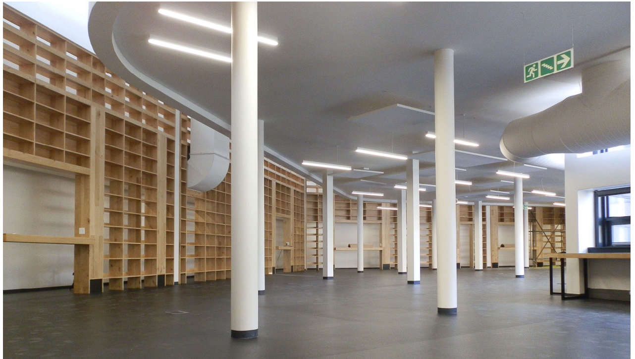
Bookracks - solid sections are the air ducts bring air to low level
